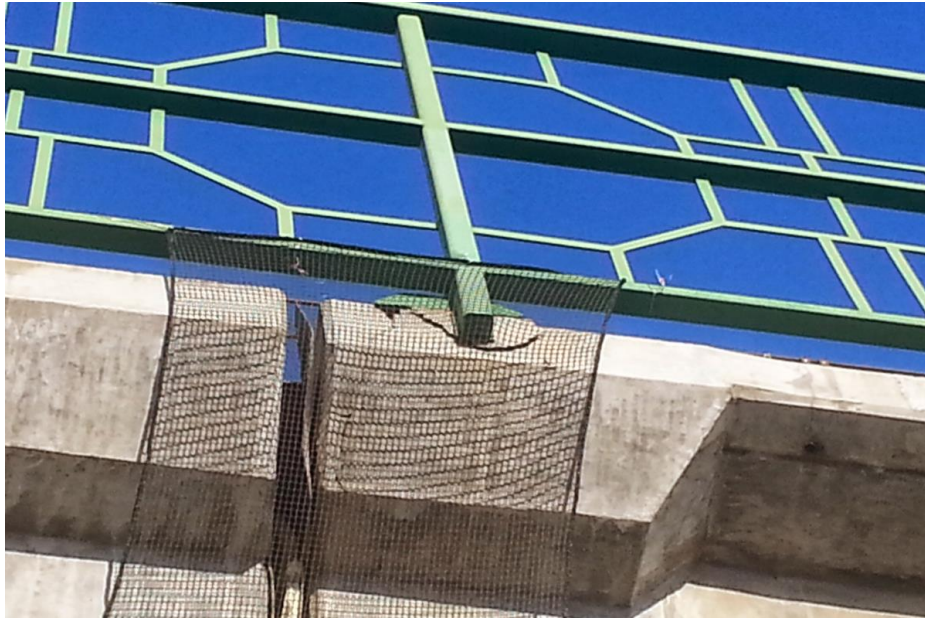
Before Repair (April 8, 2014):
