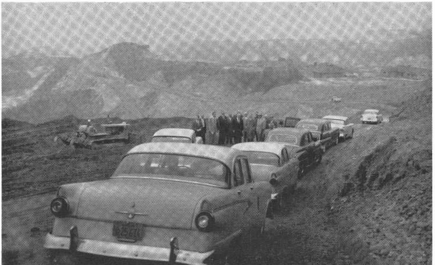
Governor's party halts on contractor's haul road to inspect work. The road is normally traveled by heavy equipment used in construction of the Ventura Freeway-San Diego Freeway interchange.
