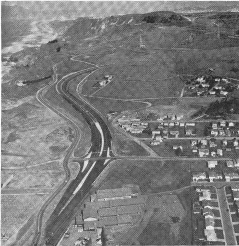
New expressway is being constructed on State Sign Route 1 between Pacifica and Skyline Boulevard just south of San Francisco. Note the old highway on the left which is benched into the bluffs to the north.
