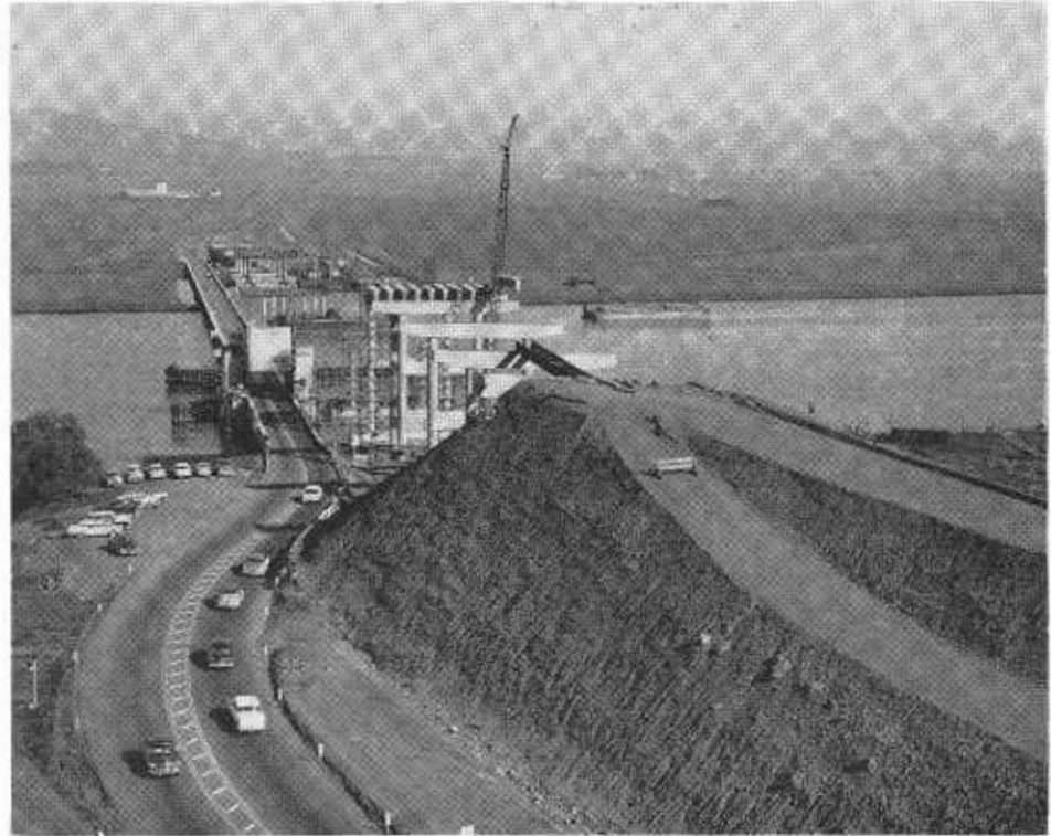
Looking east over the Petaluma Creek project. The partially completed fill in the foreground will be finished after two lanes of the new bridge are opened to traffic.
