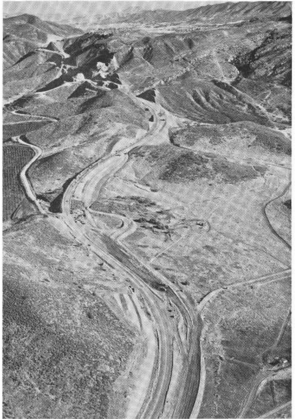
An aerial view looking east along Ventura Freeway construction on Conejo Grade. The partially completed undercrossing in the center of the picture will serve Camarillo Grove Park.
