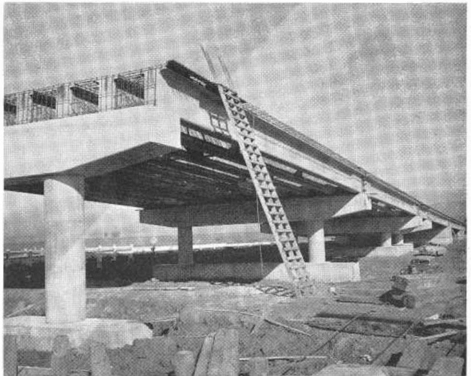
This photo of the new construction shows 80-foot, precast, prestressed girders in place on the west approach to the new bridge
