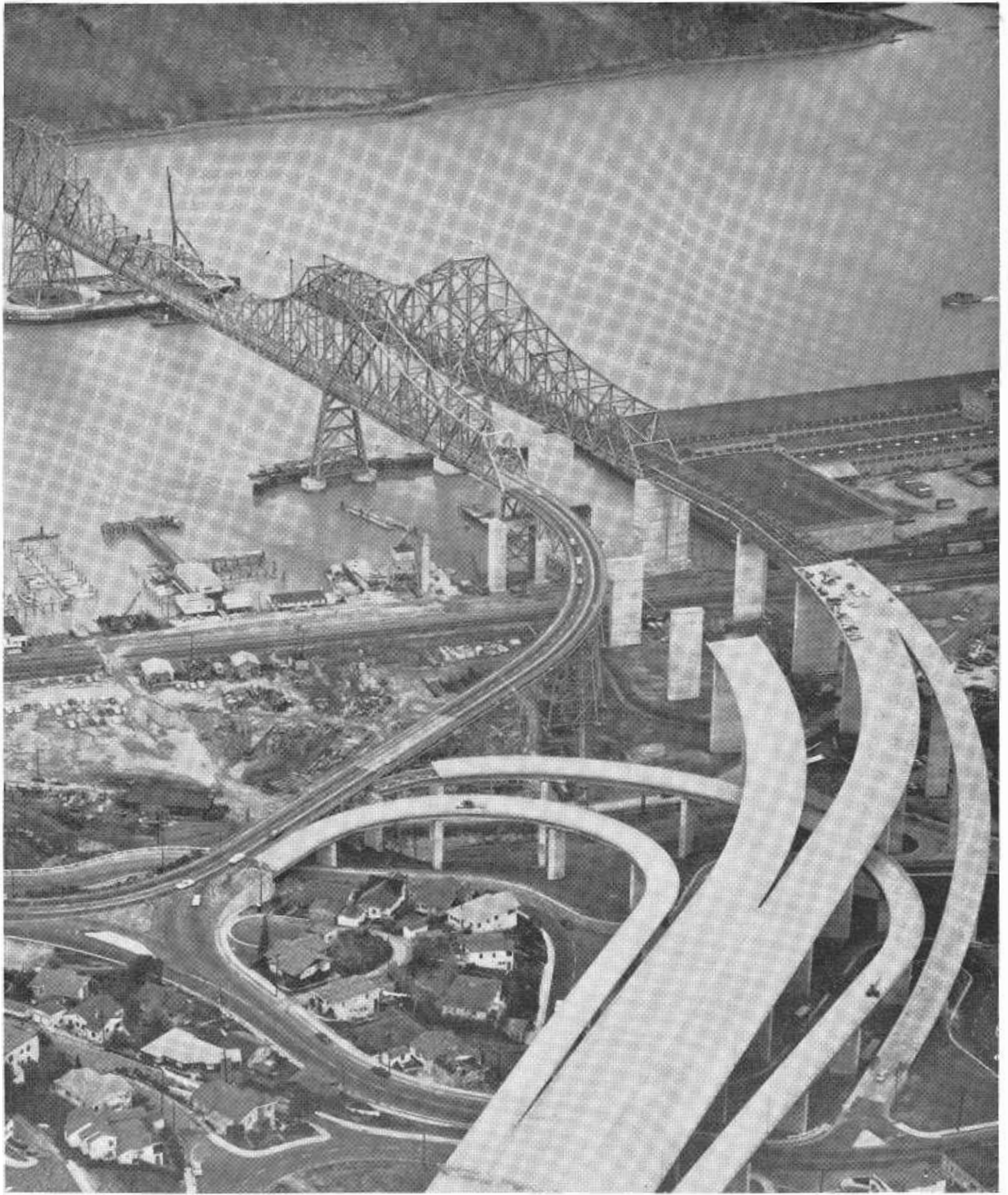
Construction on the new parallel Carquinez Bridge looking north from above the Big Cut. Crockett Interchange is in the foreground.
