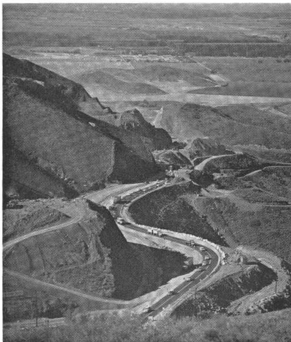
Looking west from the top of Conejo Grade showing construction in progress on the Ventura Freeway. Traffic through the construction area is being handled on a temporary detour.
