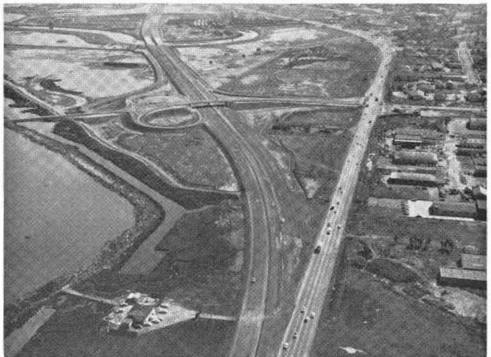
UPPER—Freeway construction on the Bayshore Freeway looking north from the San Mateo-Santa Clara County line. LOWER—Construction on the Bayshore Freeway in Redwood City. The present highway is on the right. The Whipple Avenue Interchange is on the new freeway to the left.
