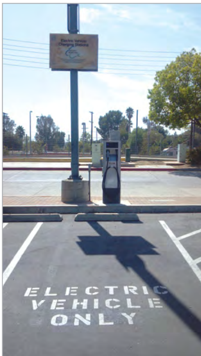
Charging slot at the Sylmar/San Fernando Station
