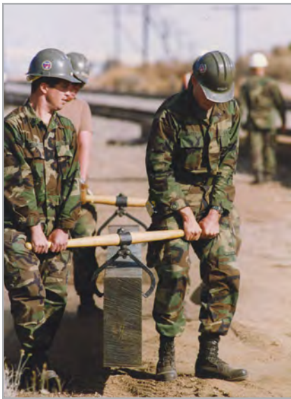
The U.S. Navy Seabees construction battalion and crews from the L.A. County Public Works quickly built the Vincent Grade/Acton Station. The station was completed in five days, compared to the usual three to six months it took to build stations at that time.
