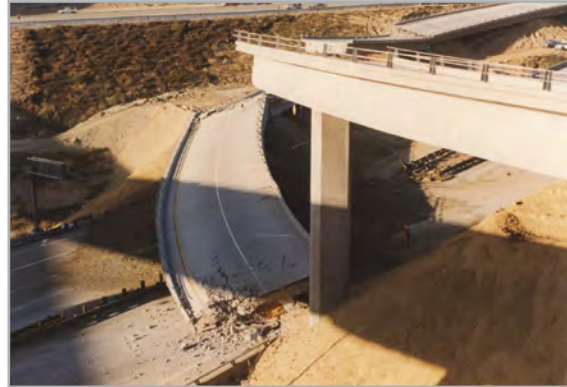
Damage caused by the Northridge earthquake
