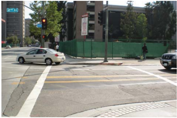
Photo 11 – The intersection of 2 nd Street and Spring Street exhibits varying degrees of infrastructure repair - potentially causing safety concerns for pedestrians and bicyclists.
