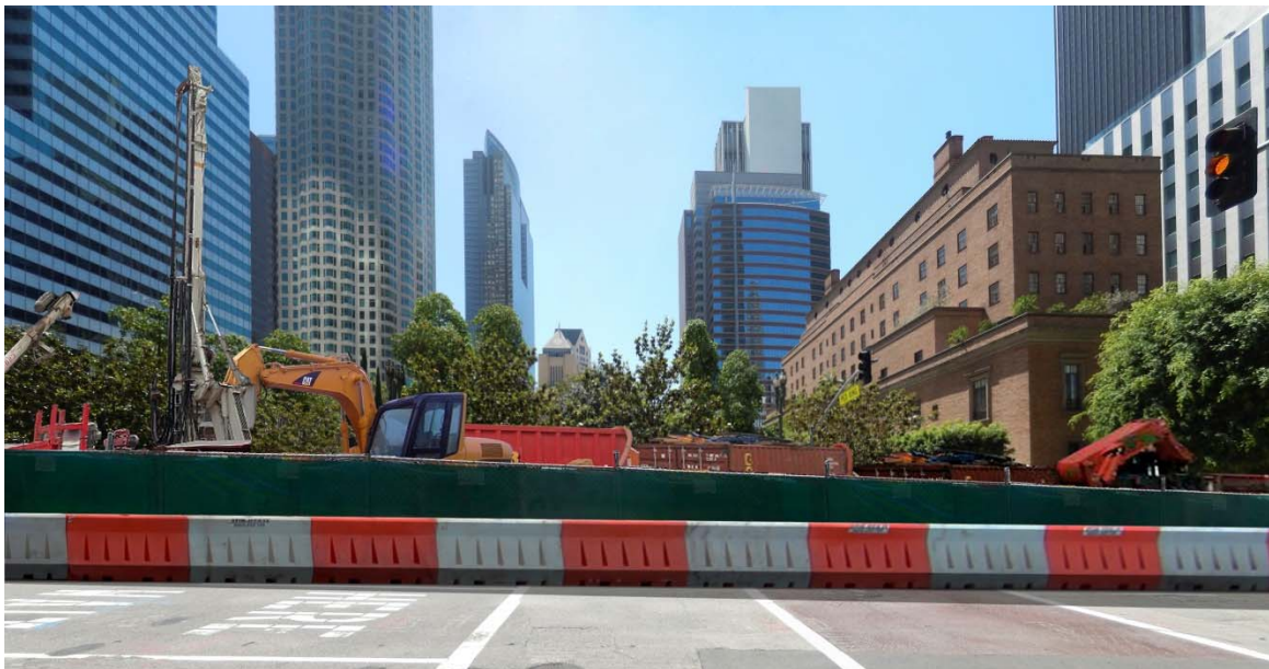
Figure 4.1-5: After View of Flower Street with Construction and Grouting Equipment Facing East Between 5th and 6th Streets
