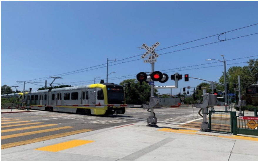
Grade Crossing Equipment on the Metro E Line
