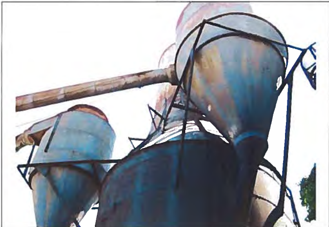
View looking northeast at attached vacuum units attached to 1957 sawdust collector.
