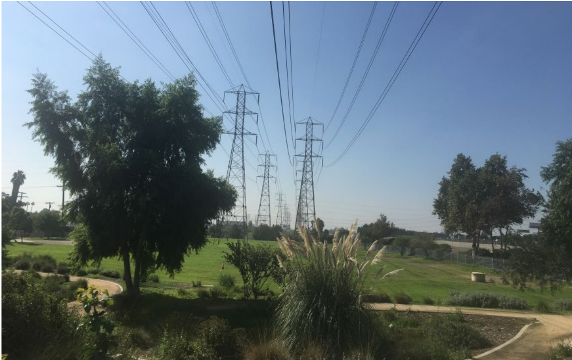
Figure 5-67. SCE's Long Beach-Laguna Bell 60kV and 220 kV Transmission Lines; Taken near their Intersection with Garfield Avenue, South-Facing
