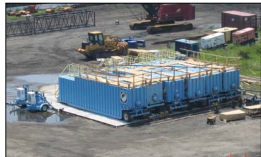
Figure 4-15: Typical Slurry Mixing Plant
