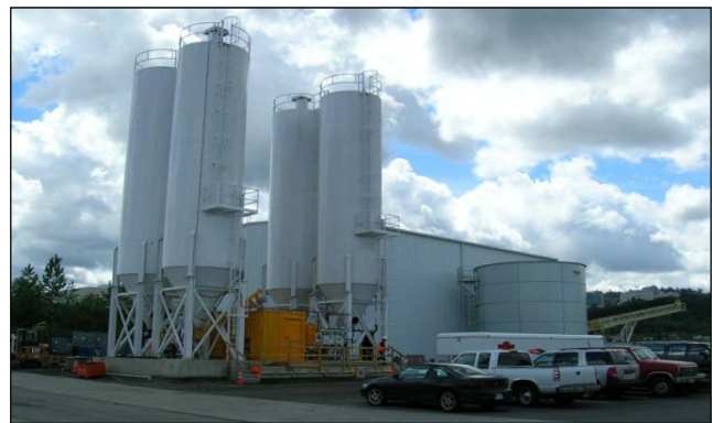
Figure 4-22: Enclosed Slurry Plant with Materials Storage Silos
