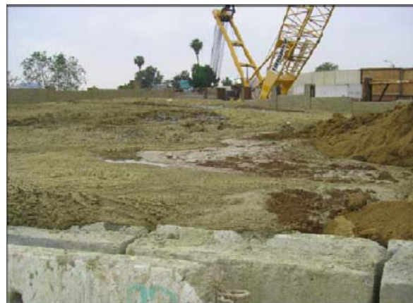
Figure 4-11: Wet Soil at Surface EPB TBM
