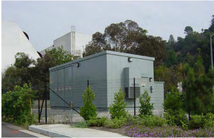
Figure 2.3-33. Typical TPSS Facility
