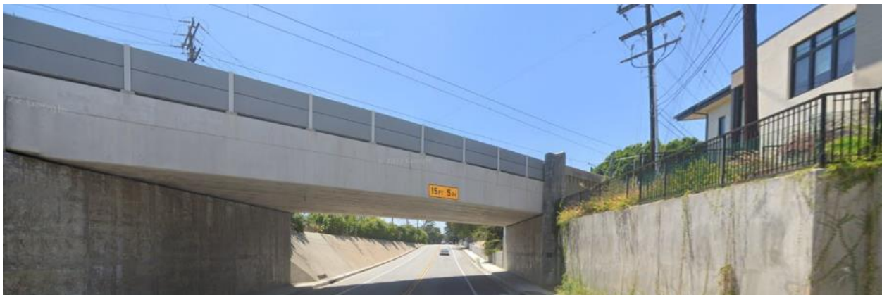
Above is one view of soundwalls on an elevated alignment of the existing Metro L Line (Gold).
