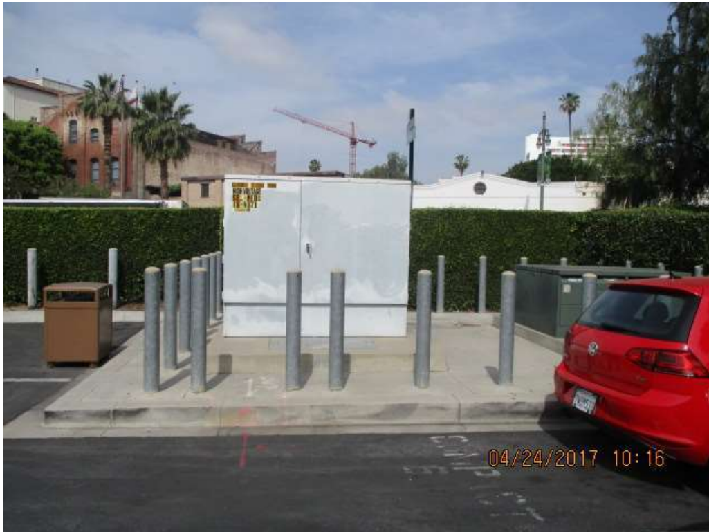
Photograph 9 - View of a pad-mounted transformer located in the northwestern portion of the LAUS Forecourt parking area.
