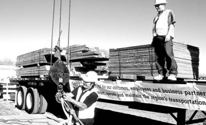
Building materials delivered to Sepulveda Basin site are being used to construct bus bridge over LA River along San Fernando Valley Metro Rapid Transitway Project.
