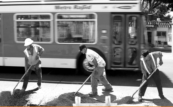
Los Angeles Department of Transportation subcontractors are as busy as ever installing Metro Rapid signal priority sensors.
