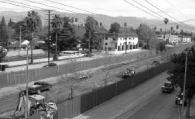
Construction of the Metro Orange Line transitway is proceeding, including the grading and paving of Chandler Boulevard between Tujunga and Whitsett avenues in North Hollywood.
