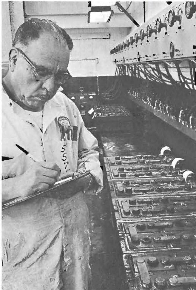
Batterymaster Pedro Perez checks batteries' performance. Units failing to meet exact specifications are sent to rebuilding firms for repair or replacement.
