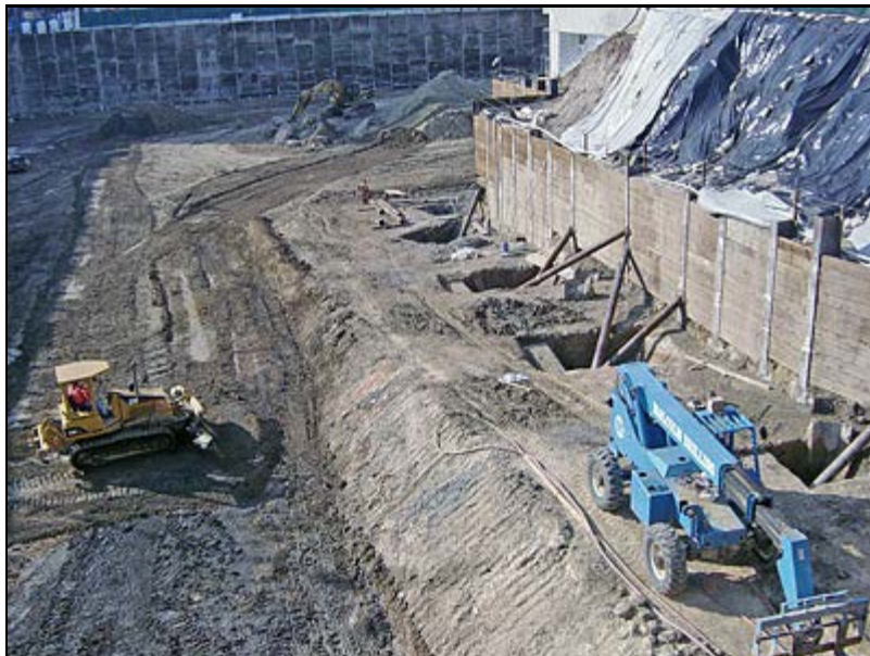
Construction machines provide a sense of the size of the construction site at Wilshire/Vermont.
