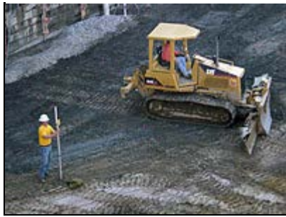
A construction worker checks a surveying instrument as a bulldozer works nearby leveling the floor of the construction site.
