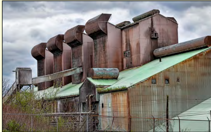
Exhibit 3-7: Weirton Steel, West Virginia. As the steel industry declined in much of the country, many mills were completely or partially abandoned, leaving behind large, often polluted sites. Because many towns were built around steel mills, these sites are often in a central location with easy rail, highway, and/or river access, making them important locations for redevelopment in many communities.
