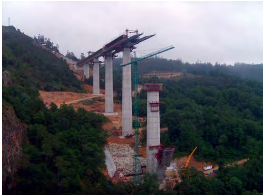
Construction of high-speed rail lines in other countries has created thousands of jobs. Here, construction is underway on a bridge as part of Spain's efforts to extend its high-speed rail network. Credit: Xosema, used under Creative Commons license
