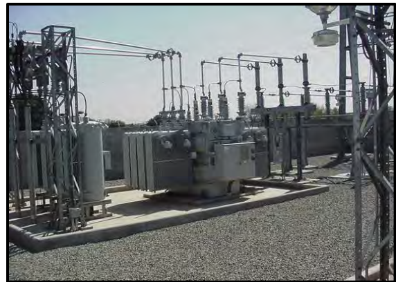
Typical Electric Substation
