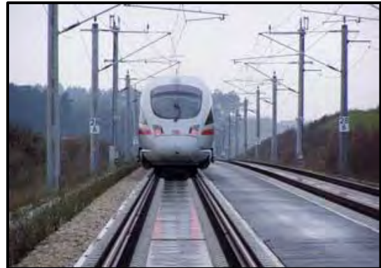
Typical Overhead Catenary
