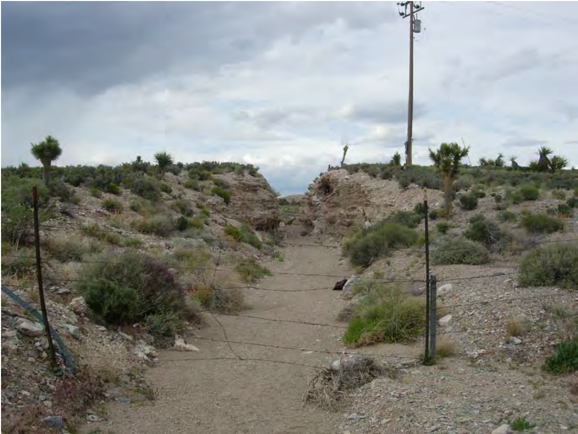
Exhibit A. Figure 17. Manmade drainage connecting to road culvert within HUC 8 Death Valley Lower Amargosa / HUC 12 Piute Valley Subwatershed
