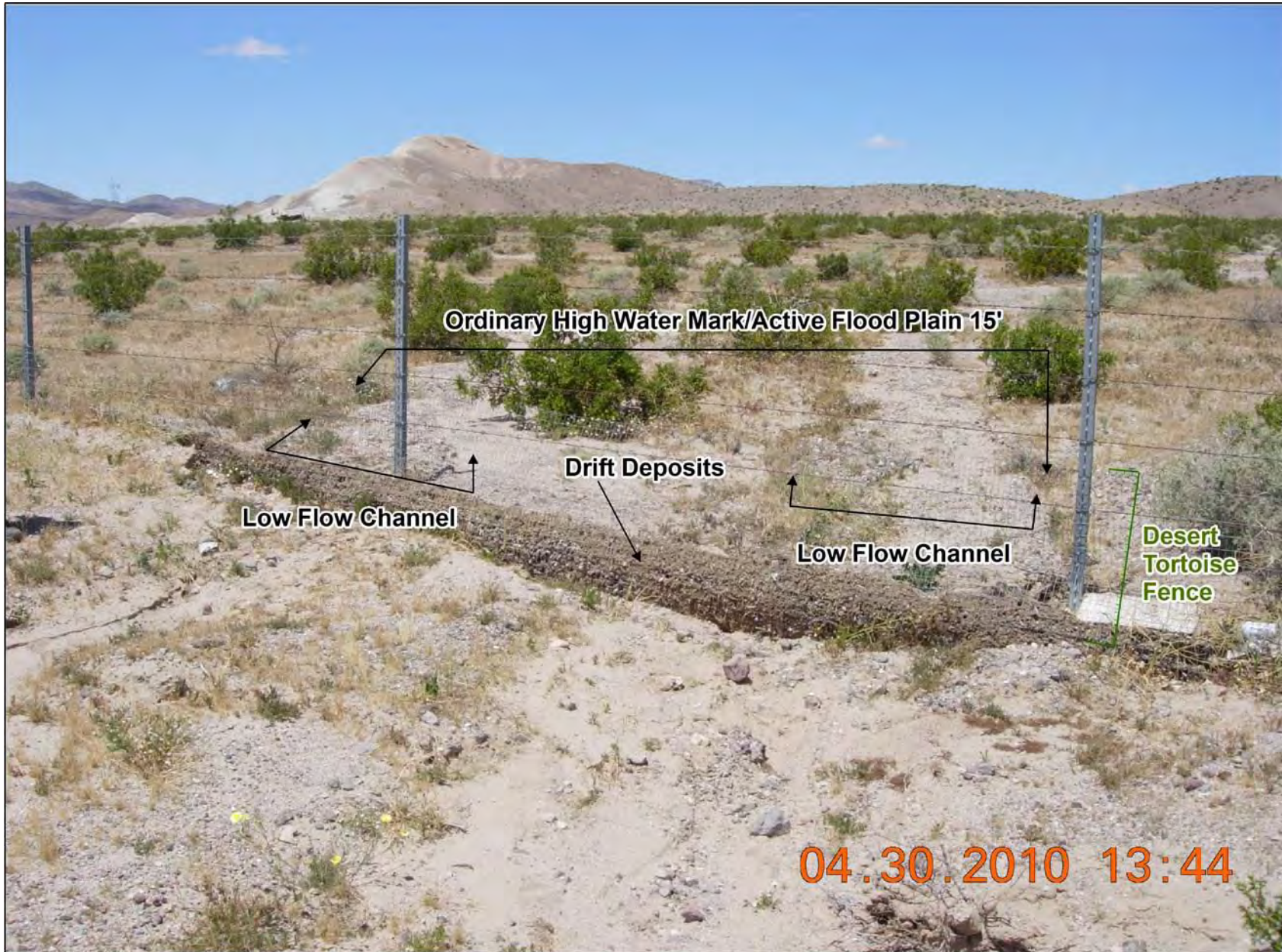
Exhibit A. Figure 11. Typical examples of field indicators of active surface water flow and Ordinary High Water Marks found within ephemerals drainages occurring within the DesertXpress Project Study Area.
