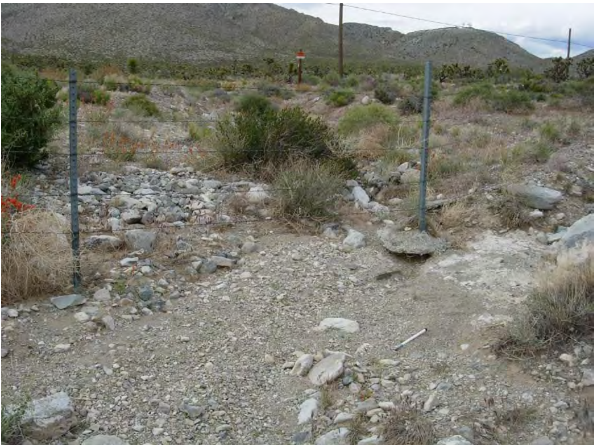
Exhibit A. Figure 18. Manmade drainage connecting to road culvert within HUC 8 Death Valley Lower Amargosa / HUC 12 Piute Valley Subwatershed
