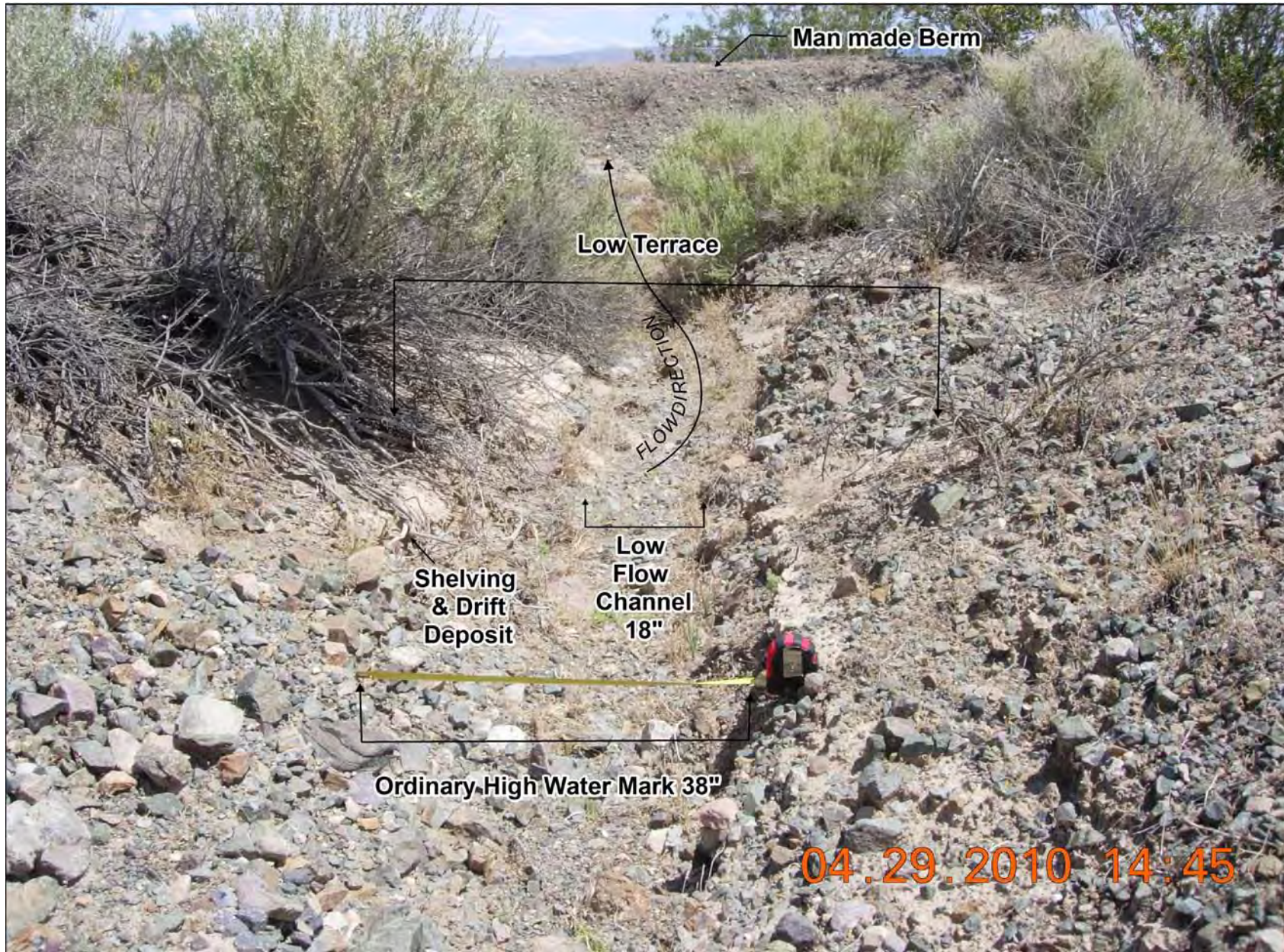
Exhibit A. Figure 8. Typical examples of field indicators of active surface water flow and Ordinary High Water Marks found within ephemerals drainages occurring within the DesertXpress Project Study Area.
