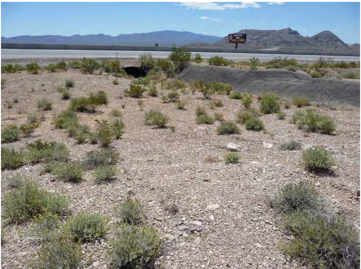
Exhibit A. Figure 28. Manmade drainage connecting to road culvert within HUC 8 Ivanpah-Pahrump Valleys Watersheds / HUC 12 Town of Jean -Frontal Ivanpah Lake Subwatershed
