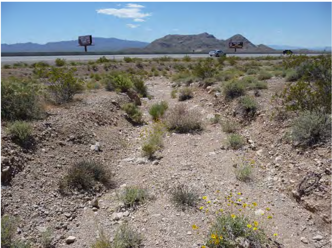
Exhibit A. Figure 32. Manmade drainage connecting to road culvert within HUC 8 Ivanpah-Pahrump Valleys Watersheds / HUC 12 Town of Jean -Frontal Ivanpah Lake Subwatershed
