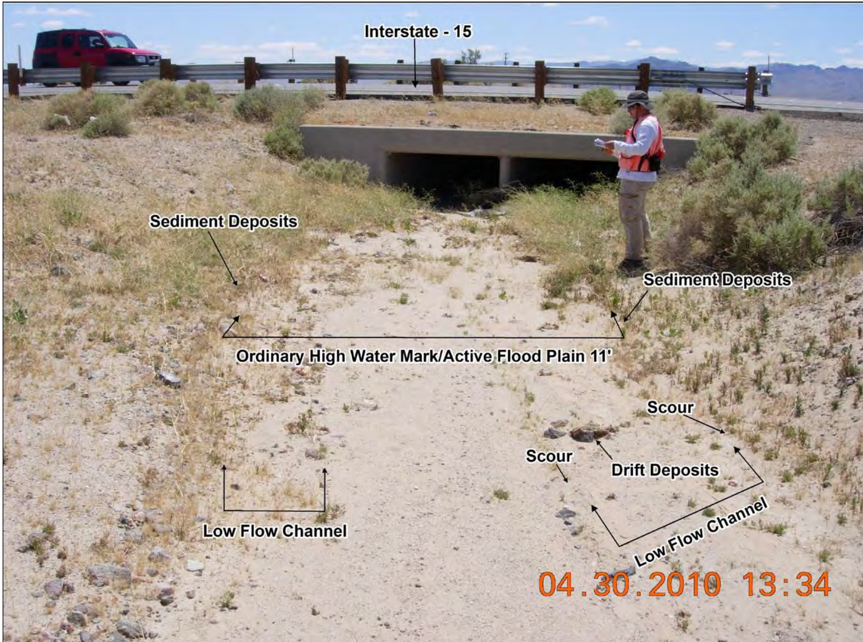
Exhibit A. Figure 12. Typical examples of field indicators of active surface water flow and Ordinary High Water Marks found within ephemerals drainages occurring within the DesertXpress Project Study Area.
