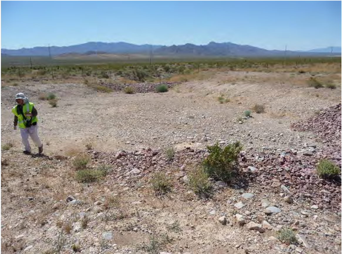
Exhibit A. Figure 13. Manmade drainage connecting to road culvert within HUC 8 Ivanpah-Pahrump Valleys Watersheds / HUC 12 Ivanpah Subwatershed
