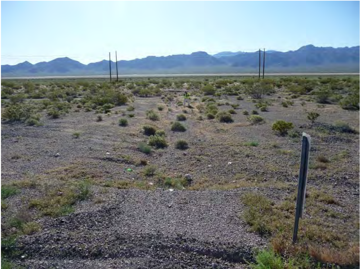
Exhibit A. Figure 21. Ephemeral drainage connecting to road culvert within HUC 8 Ivanpah-Pahrump Valleys Watersheds / HUC 12 Porter Wash -Frontal Ivanpah Lake Subwatershed
