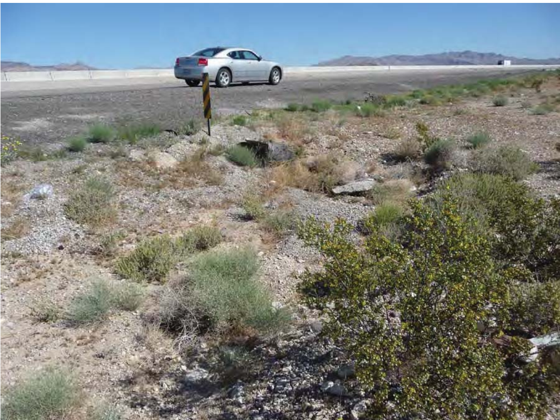
Exhibit A. Figure 18. Manmade drainage connecting to road culvert within HUC 8 Ivanpah-Pahrump Valleys Watersheds / HUC 12 Porter Wash -Frontal Ivanpah Lake Subwatershed
