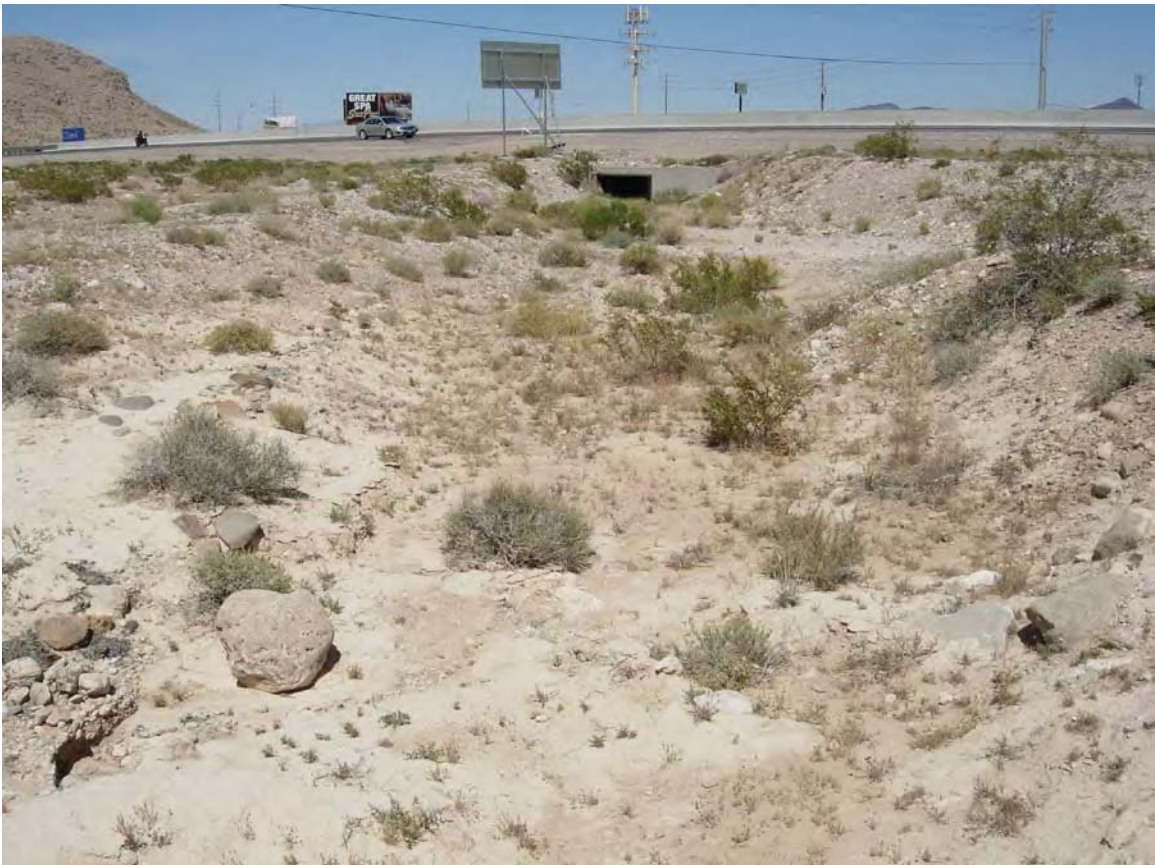
Exhibit A. Figure 16. Manmade drainage connecting to road culvert within HUC 8 Las Vegas Wash Watershed / HUC 12 Town of Sloan Subwatershed
