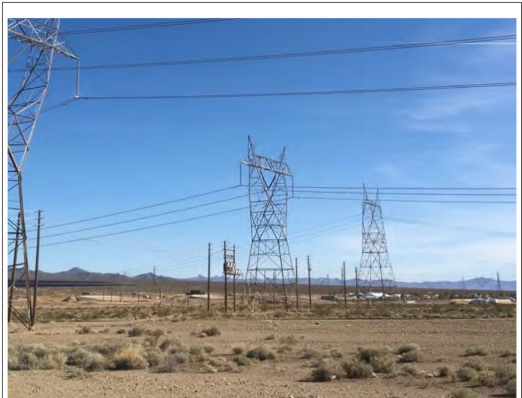
Los Angeles Bureau of Power and Light Boulder Line 2 (mid
