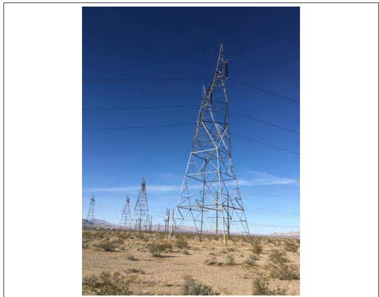
Los Angeles Bureau of Power and Light Boulder Line 1 (fore
