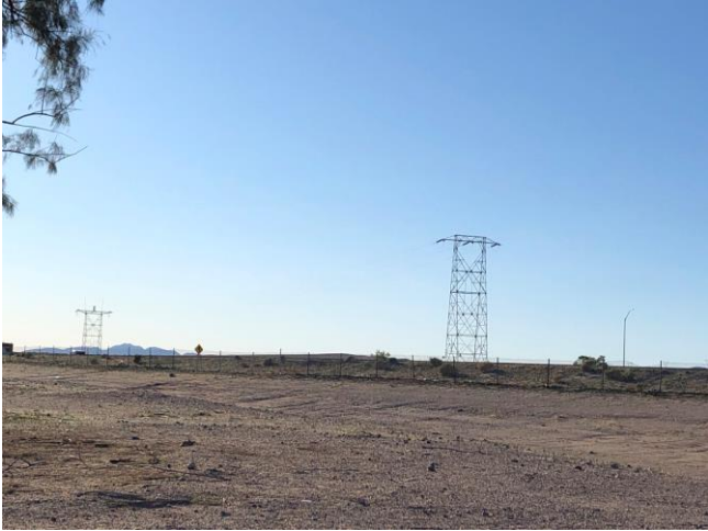
Segment 5, east end, north side. Type A dead-end tower (right), Type SW Tower (left), camera facing west
