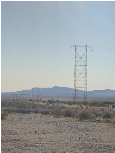
Segment 5 at Field Road, north side. Type A dead-end tower (left, foreground), Type H tower (left, background), camera facing southwest
