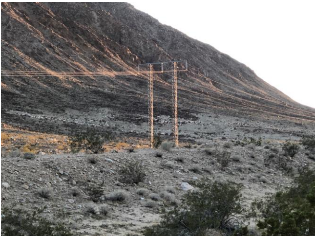
Segment 4, east end, south side. Standard Type H tower, camera facing southwest
