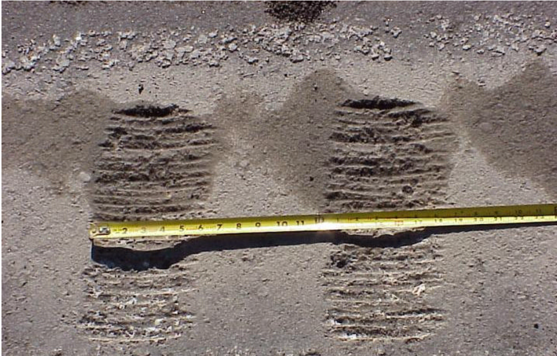
Figure 5. One of the shallower sections of standard rumble strip. The grooves are on 12-inch centers. The wear on the grinder teeth is shown by the uneven shape and variation in depth along the grooves.
