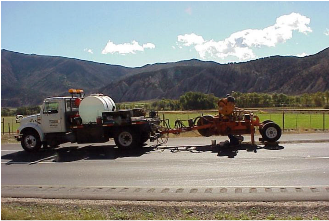
Figure 3. The equipment used to grind the standard rumble strips. The operation is stopped and the trailer raised so the operator can replace worn teeth on the grinding drum.
