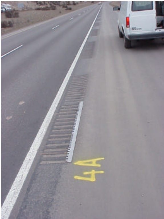
Figure A-12. Section 4A is ground in an interrupted pattern using the same spacing as section 4 – 2-inch grooves, ½ inch deep, with 3-inch flats.
