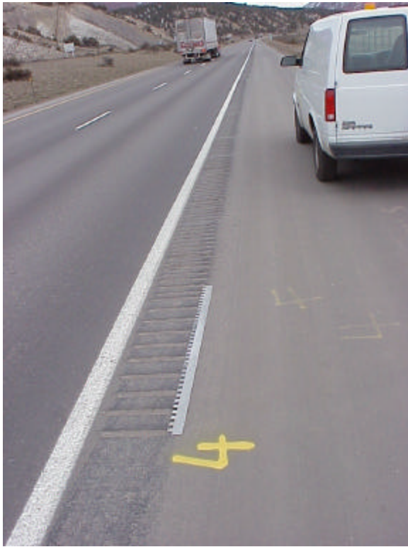
Figure A-11. Section 4 starts at the far end of the straight edge. Grooves are 2 inches wide but with only 3-inch flats between. Section 4 is continuous rumble strip.
