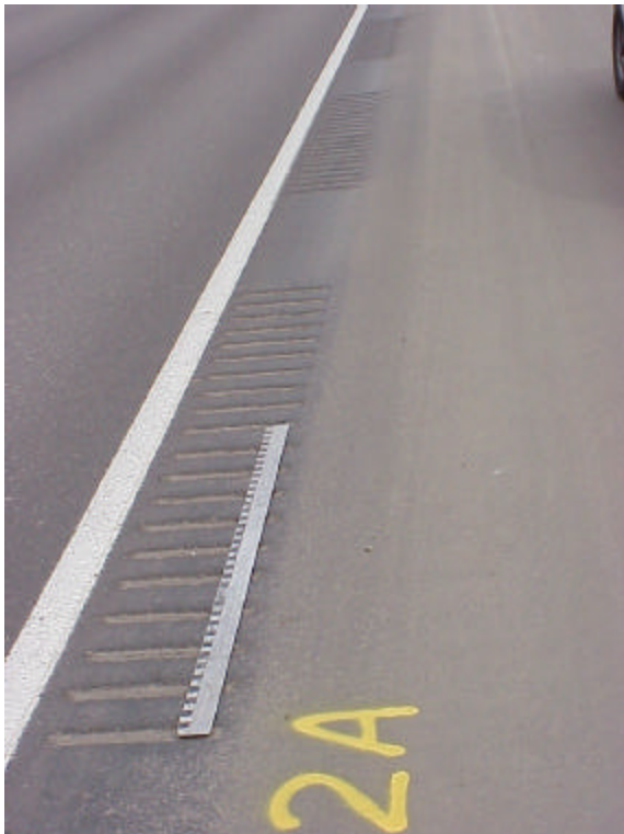
Figure A-8. Section 2A, like sections 1A and 4A, is interrupted every 12 feet. The grooves are 2 inches wide with 5-inch flats, and were ground \frac{1}{2} inch deep.
