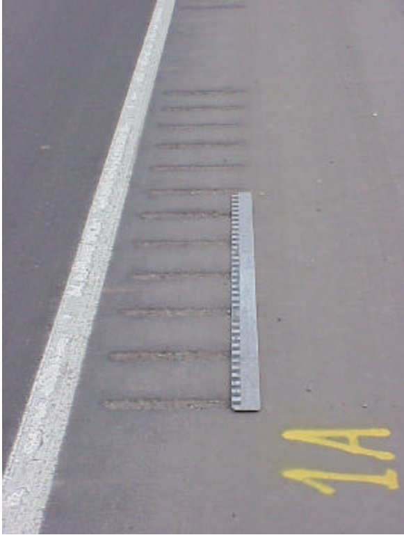
Figure A-5. Spacing for sections 1 and 1A were the same. The only difference was that the rumble strip was ground with gaps for section 1A. For every 12 feet of rumble strip, a six- foot gap with no grooves was left.
