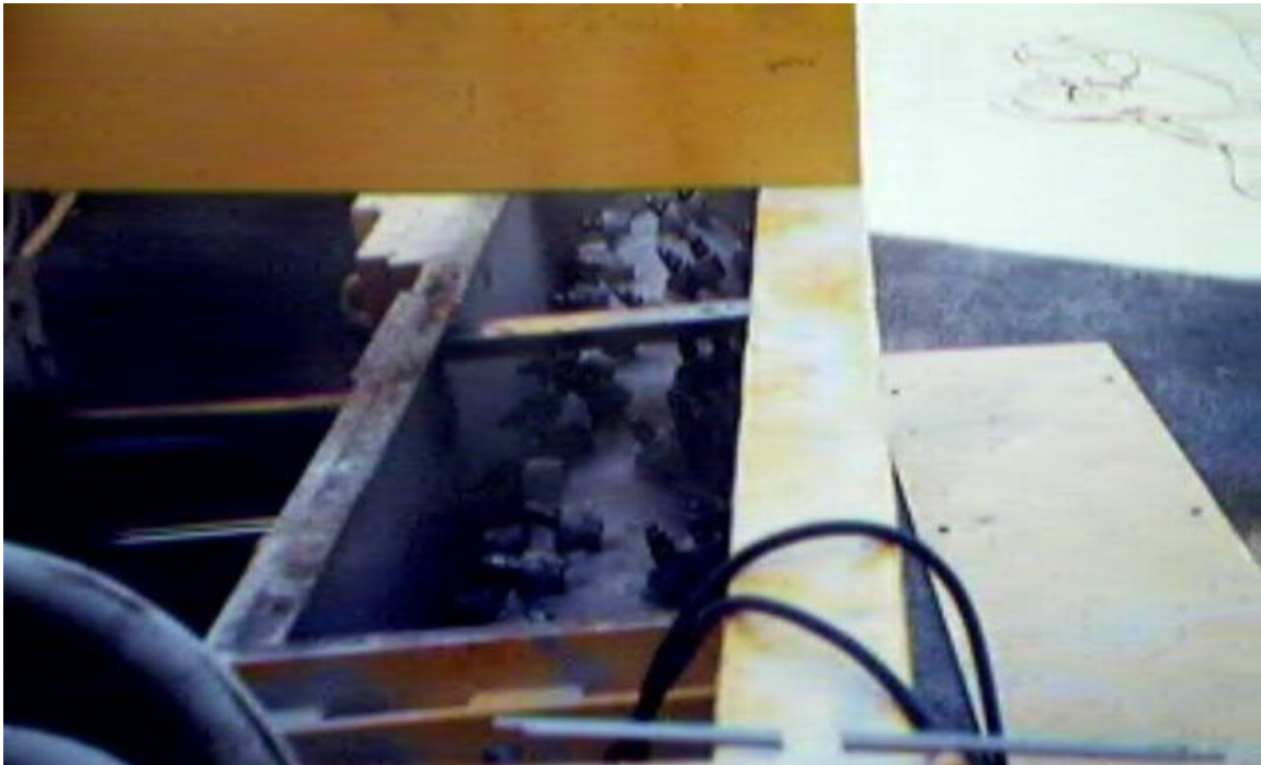
Figure 11. The grinding drum on the new two-inch-groove machine. The spaces between the sets of teeth that adjusts the spacing of the grooves can be seen. The spinning drum is lowered into the pavement and moved to the left to cut the rumble strip grooves - six feet at a time.
