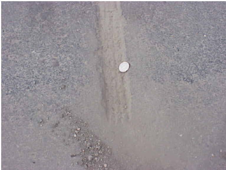
Figure A-4. The uneven bottom of the groove in this picture shows where the teeth on the grinder drum cut the asphalt. A quarter is leaning against the side of the groove for a rough size comparison. This groove was full of dirt and sand like the one above but the debris was swept out before the picture was taken.
