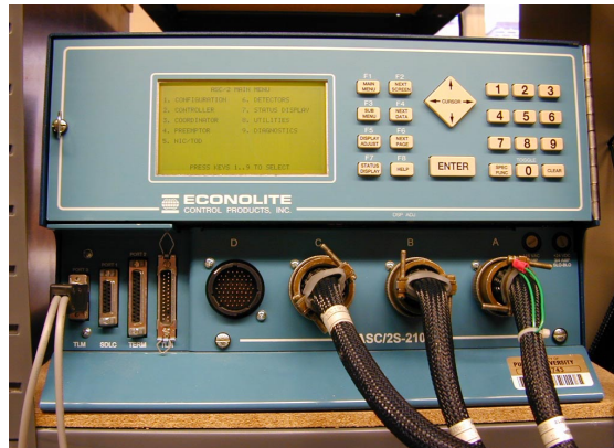
(a) Local Controller
