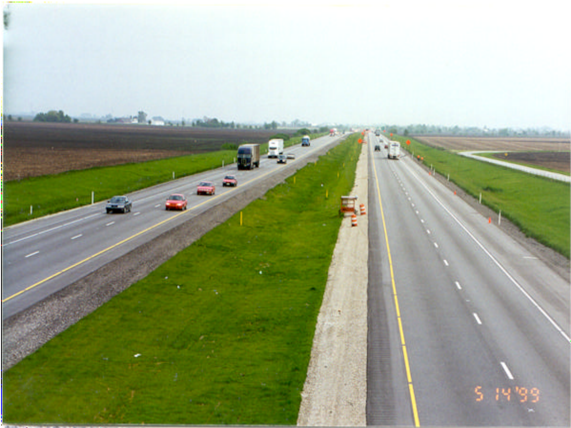
Figure 5.1: Southbound side of the construction zone (MP 180 near US 43 interchange) view from CR 800S overpass
