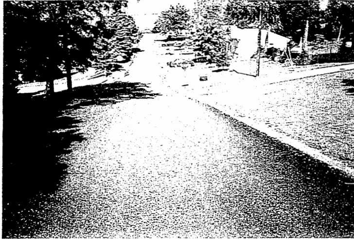
Figure 29. Oak Hill Drive - Centerline viewed from approach to curve in the 2 nd half of the test section, looking downhill toward North View Court and beginning of test section.
