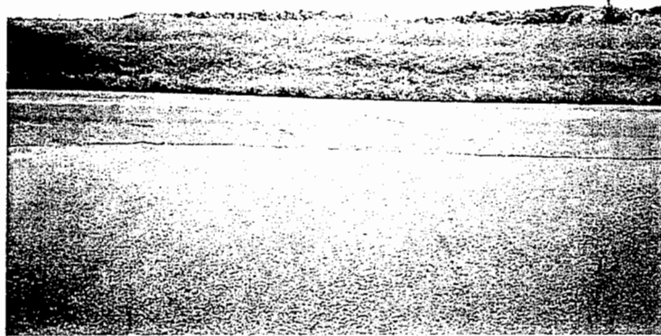
Figure 25. Wheat truck damage to FB-3 Modified on Rinely Road at Clark Road intersection as viewed from Clark Road.
