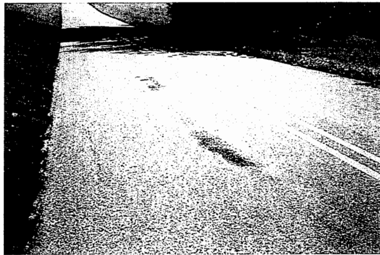
Figure 24. Rinely Road test section 1 - Original reflection crack and chip seal binder that has migrated up to FB-3 surface.
