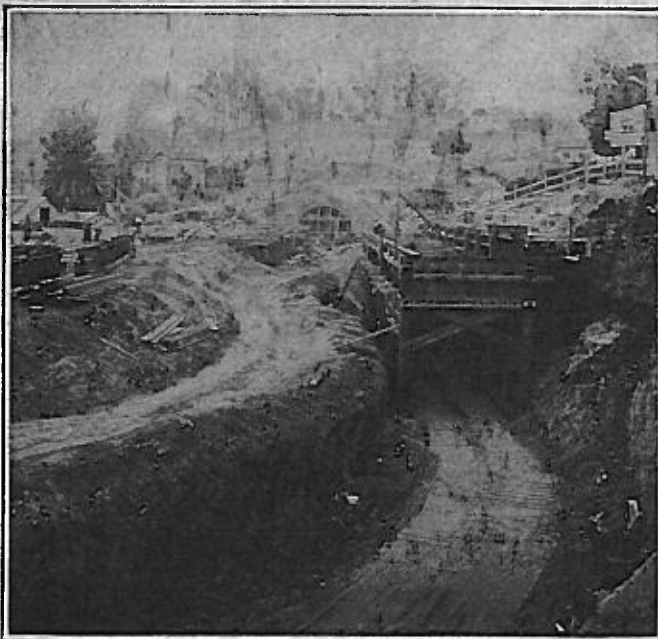
In Digging the New Los Angeles Subway, Excavated Material Is Removed by a Light Railway and Dumped Into Timber Bunkers, from Which It Is Hauled Away by Motor Trucks
