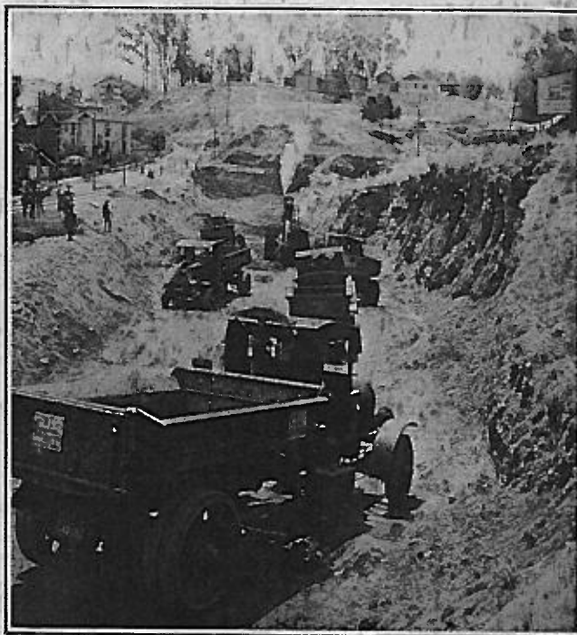
Beginning the Excavation at the West Portal of the New Hollywood-Glendale Tunnel in Los Angeles
