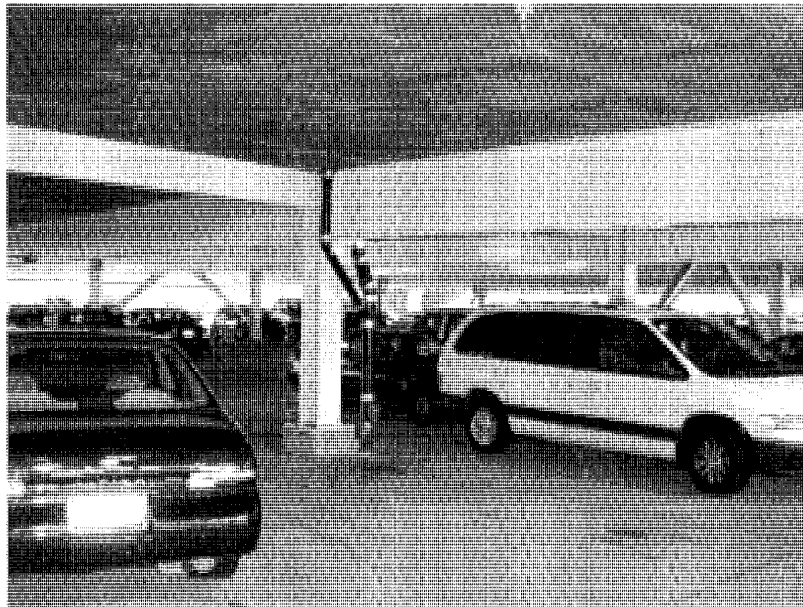
Interior view of steel framed parking structure with braced frames, but no shear walls.
