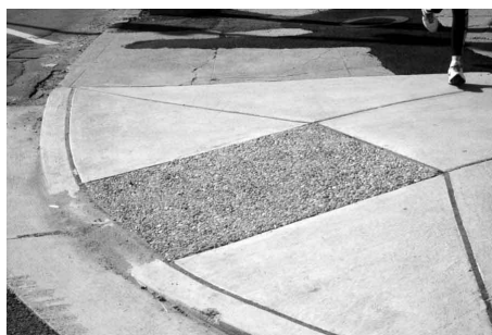
FIG. 5-2. CURB RAMP EXPOSED AGGREGATE SURFACE IN VIRGINIA. PEDESTRIANS WHO ARE BLIND DO NOT RELIABLY DETECT EXPOSED AGGREGATE CONCRETE.
