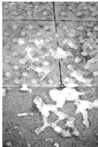
FIG. 5-5. DETECTABLE WARNING SURFACE WITH A PARTIAL SNOW COVER BETWEEN THE DOMES, ANCHORAGE, ALASKA.
