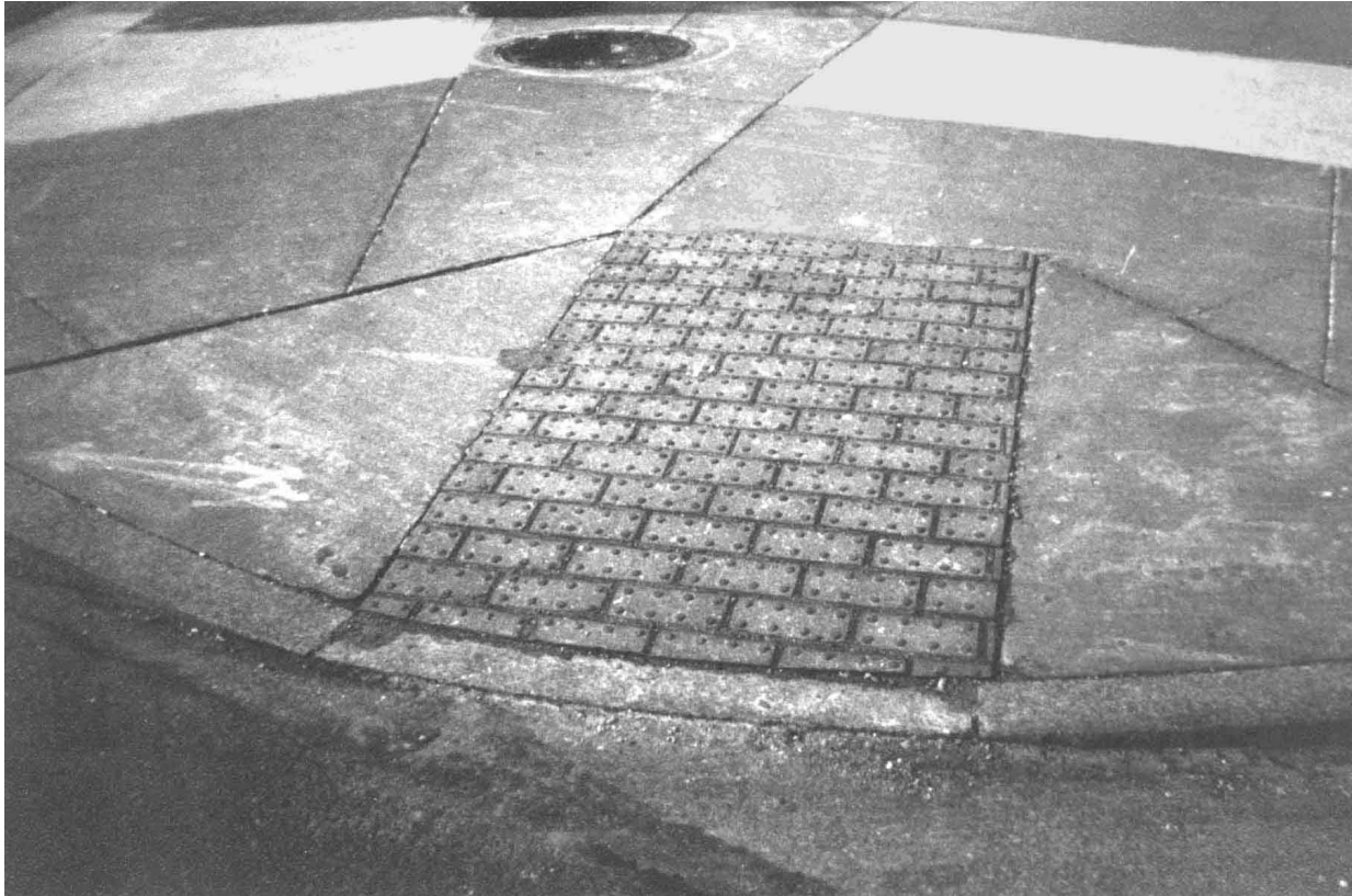
FIG. 0-2. CURB RAMP COMPLYING WITH ADAAG 4.7.7 (TEMPORARILY SUSPENDED), CLEVELAND, OH.
