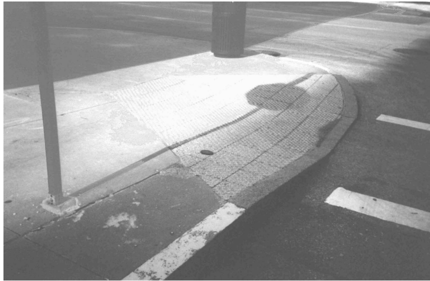
FIG. 5-13. TRUNCATED DOME PAVERS CUT AND FITTED TO THE ENTIRE SURFACE OF A PERPEN- DICULAR CURB RAMP, INCLUDING FLARES, CLEVELAND, OH.
