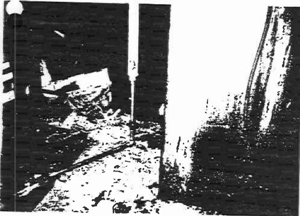
DEBRIS ON FLOOR OF BOILER ROOM NEXT TO HOT WATER TANK
