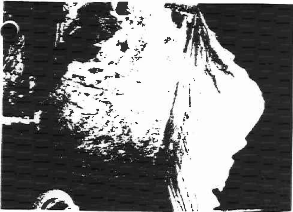
CLOTH DAMAGE A7 MAIN EXHAUST DUCT BOILER ROOM
