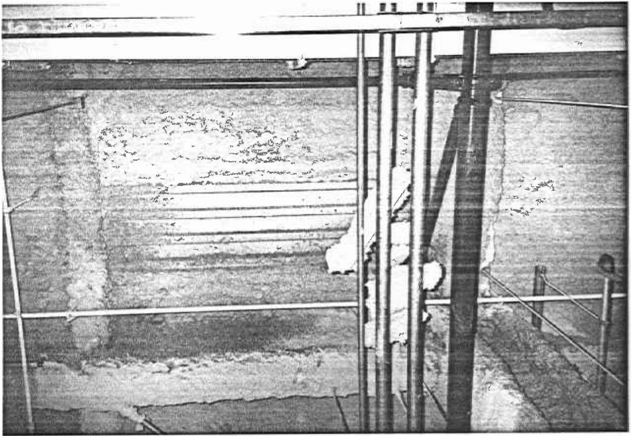
RM. 249-- EXPOSED ROOF DECK W/ FIREPROOFING MISSING.
