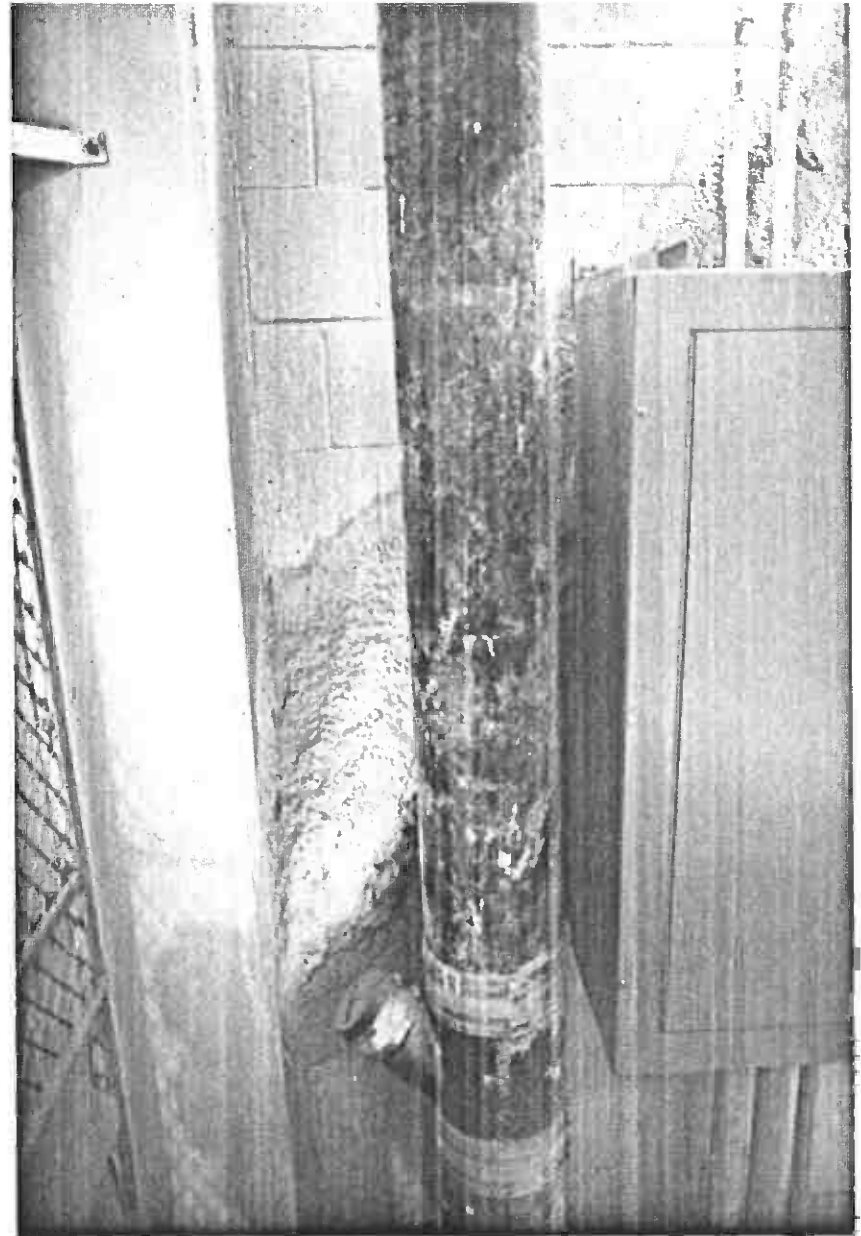
RM. 134- COL. G-18 BRACE BEHIND DRAIN LINE
