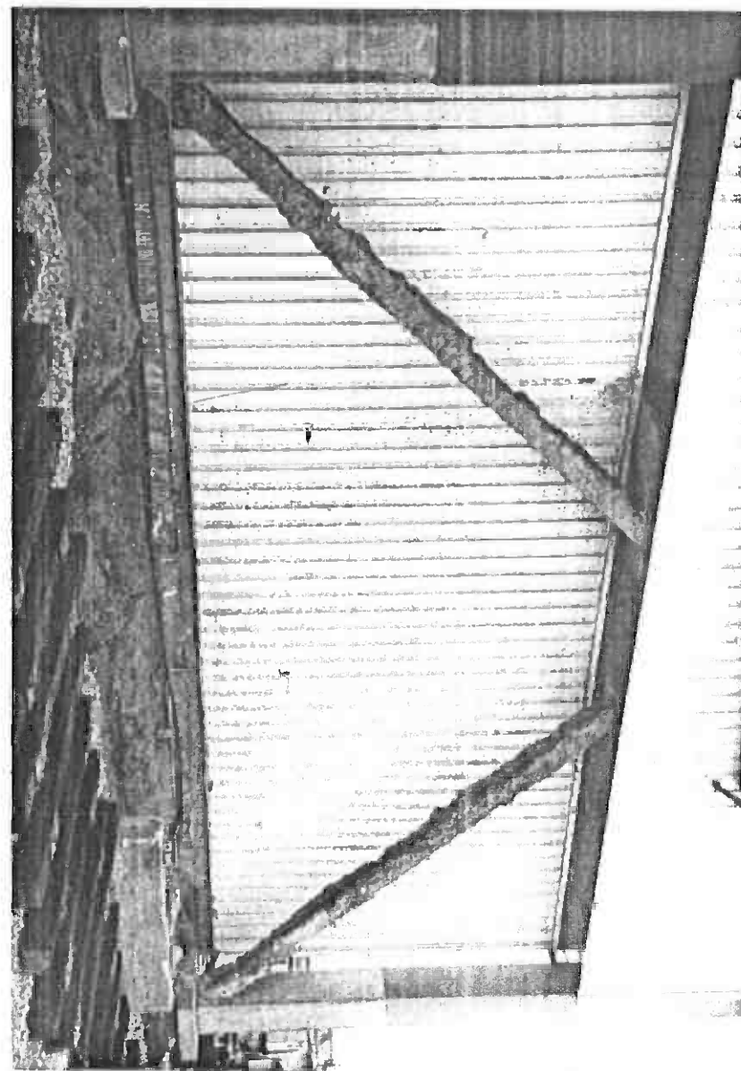
EXTERIOR K-BRACE AT GRIDLINE 1A
