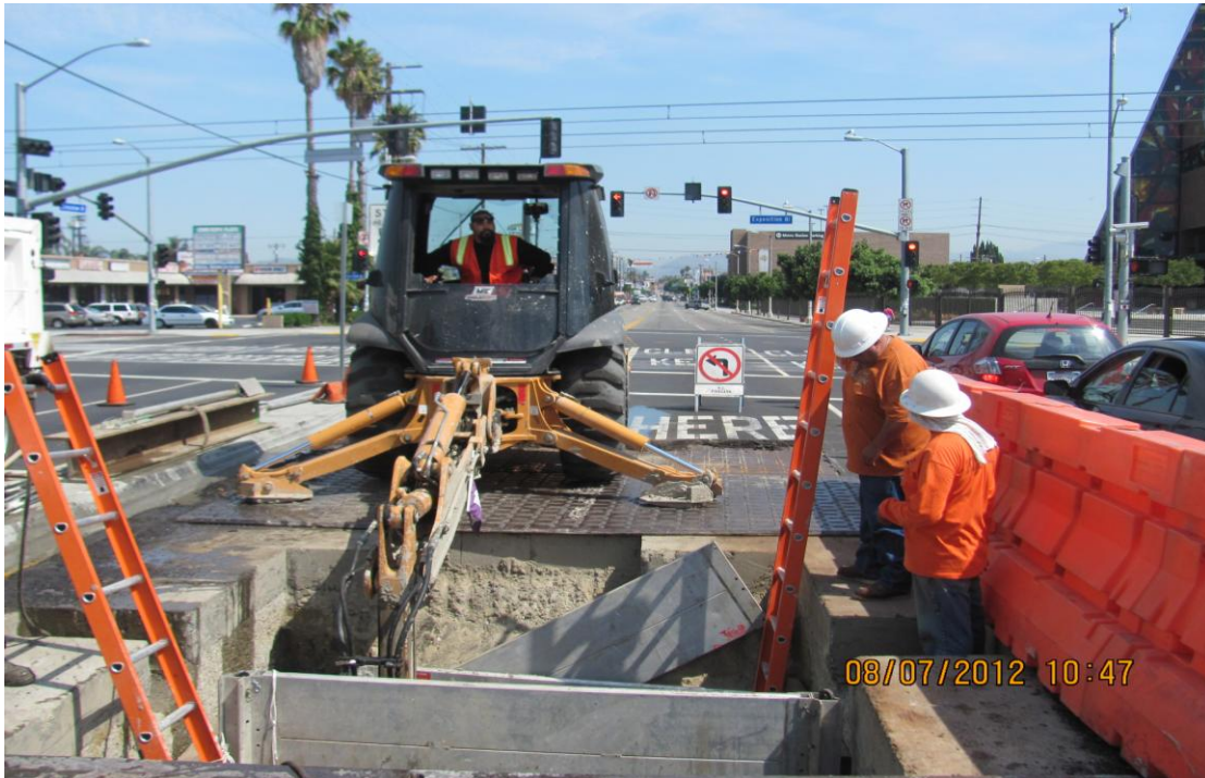
Southern California Gas Co. advance relocation of gas line at Crenshaw Blvd. and Exposition Blvd.
