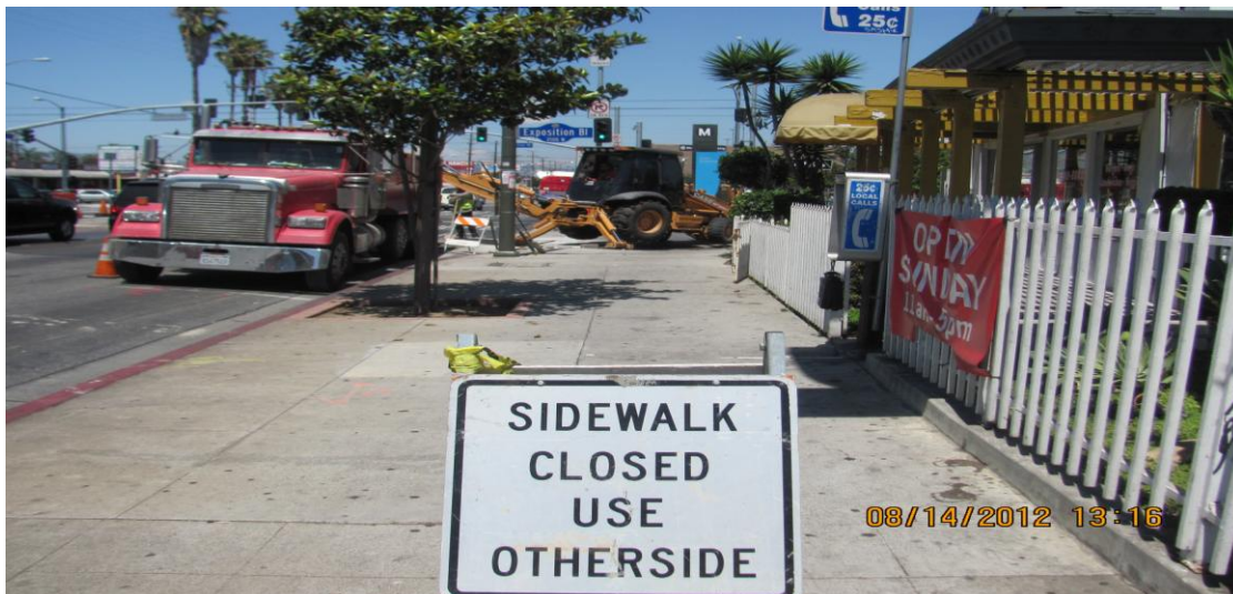
Southern California Gas Co. advance relocation of gas line at Crenshaw Blvd. and Rodeo Rd.
