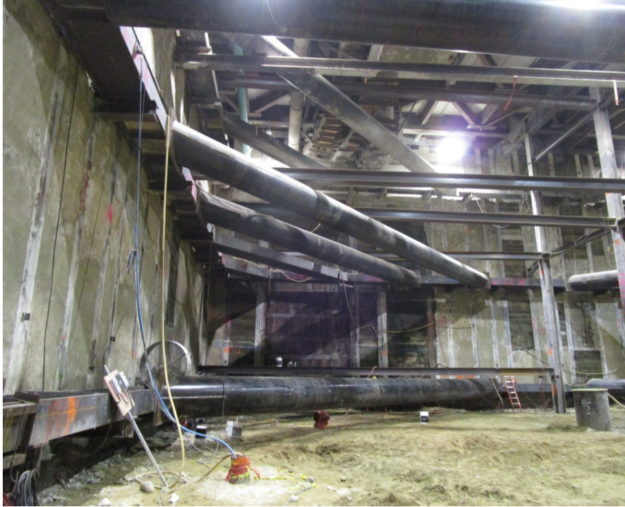
EXPOSITION STATION – Tier 3 excavation in the north-west portion of the north station box.
