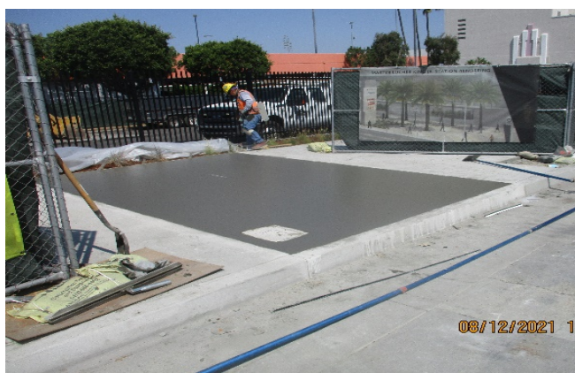
MLK STATION SITE – Placed concrete for sidewalk panel on southbound Crenshaw Blvd between Stocker St and Martine Luther King Blvd.
