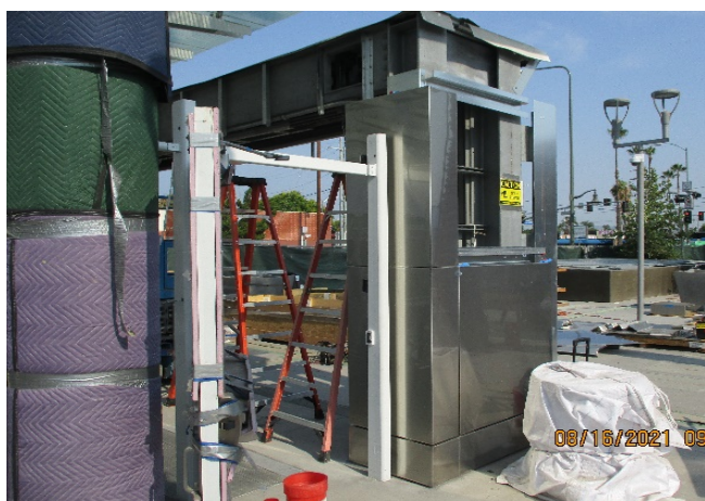
EXPO STATION – Continue stainless steel cladding panel installation to the main entrance roll-up door.
