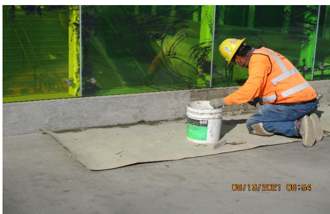
LEIMERT PARK STATION – Sacking and patching the concrete curb around the main entrance plaza canopy.
