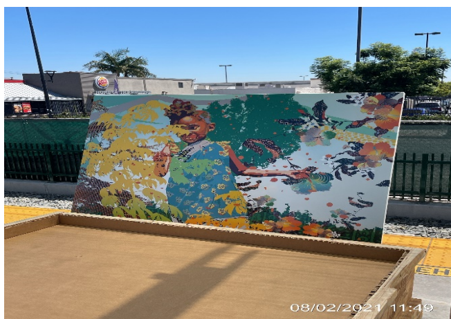
HYDE PARK STATION – Delivered and prepared for porcelain enamel steel art panel installation.
