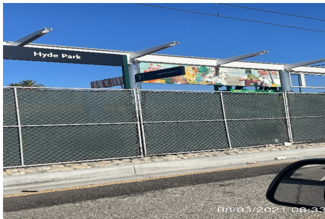
HYDE PARK STATION – Installing porcelain enamel steel art panel along the entire center canopy at the platform.
