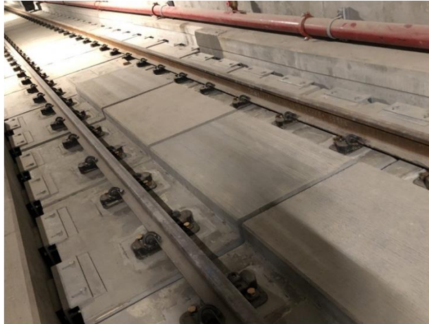
DF Track assembled in left tunnel Reach 2
