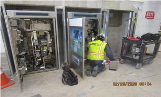
Leimert Park Station – Continue installing and wiring the ticket vending Machines at the Free Area.
