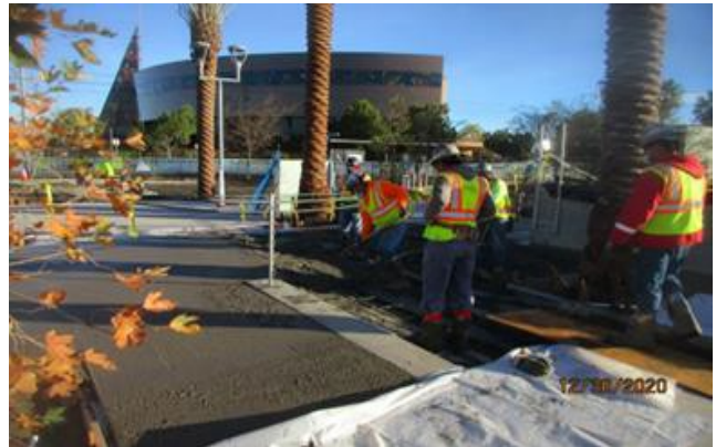
Expo Station – Continue placing concrete for the architectural topping slab at the north side of the plaza.
