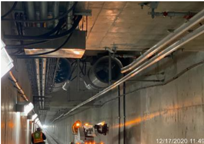
UG3- Start-up crew inspecting fans in tunnel.
