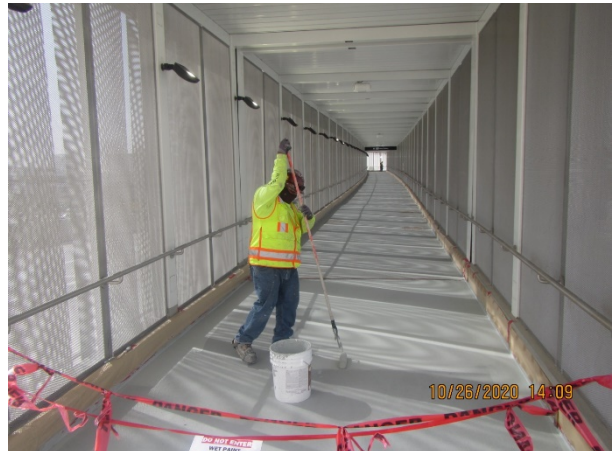
Pedestrian Bridge Punchlist
