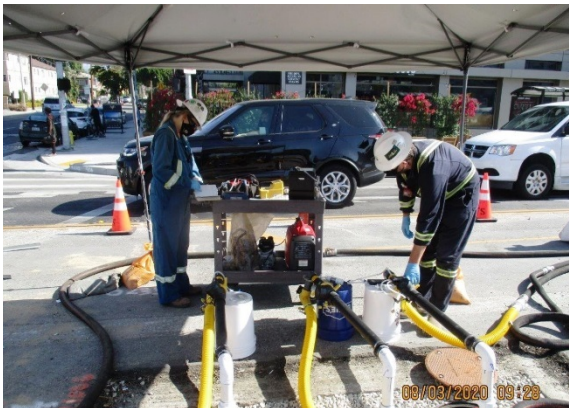
Reach 3 Gas Extraction
