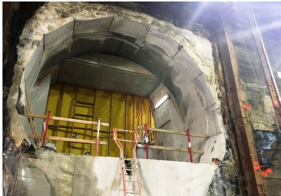
Wilshire/Western Interface Chamber
