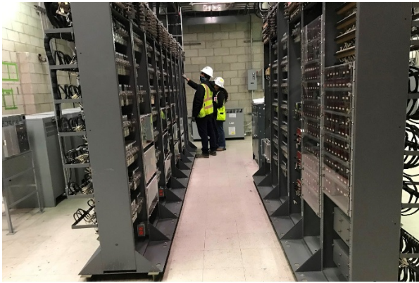
Inside TCC Room at Wilshire/Western Station
