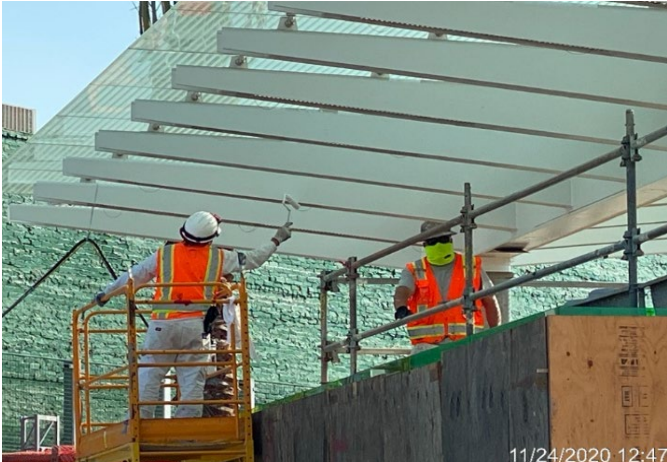
Leimert Park Station – Applying finishing paint to main entrance canopy outriggers at plaza level.
