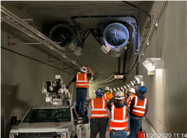
UG4- Testing and inspection of tunnel booster fans in preparation for start-up-energization.
