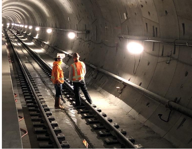
LVT Blocks and rail in Reach 1 right tunnel
