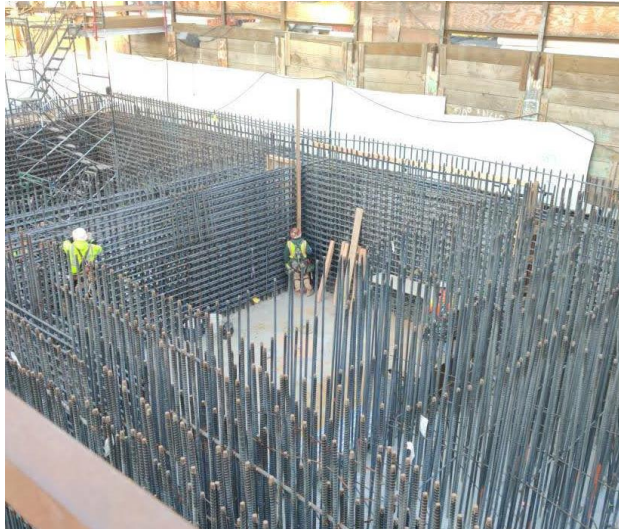
Entrance Roof stem walls formwork and rebar in progress at Historic Broadway Station
