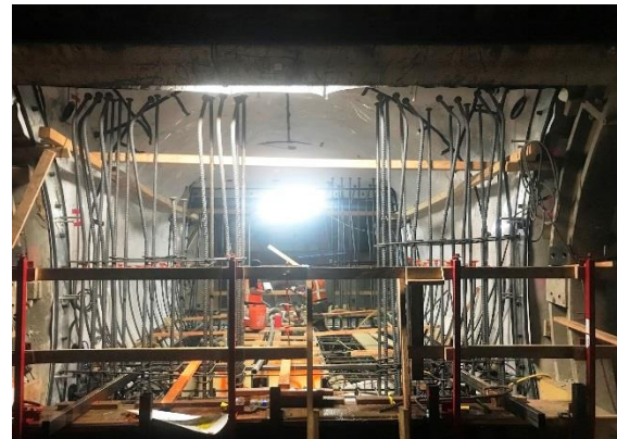
Cross Passage #14 (Reach 1) Electrical Installation
