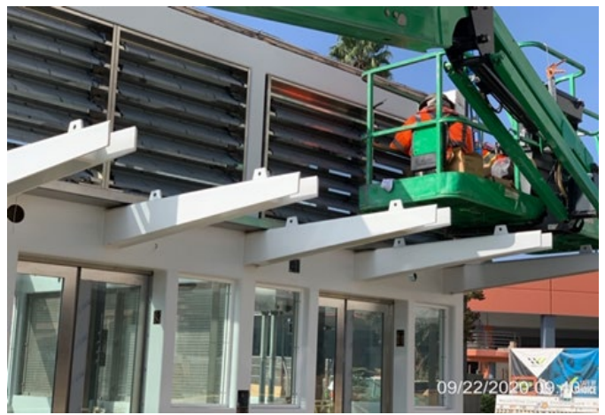
Martin Luther King Jr. Station – Continue installing louvers and gutters to elevators 1 & 2 at the plaza level
