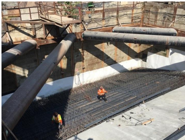
Rebar installation at Roof Level deck at Grand Av Arts/Bunker Hill Station
