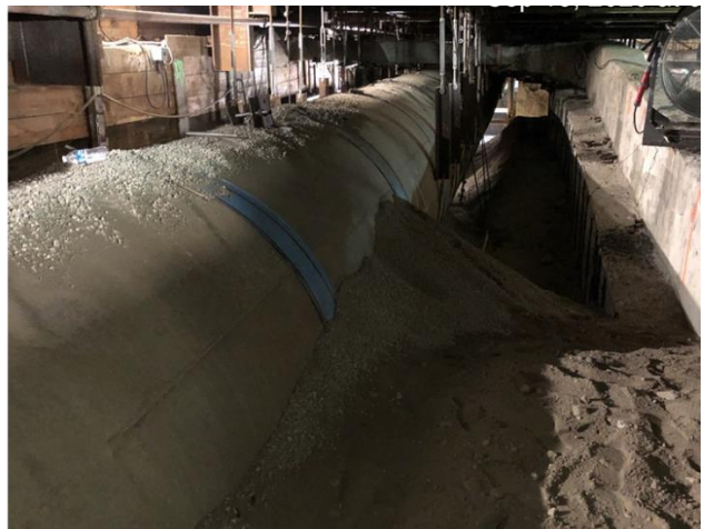
Backfill east and west of 72-inch RCP storm drain under Flower St
