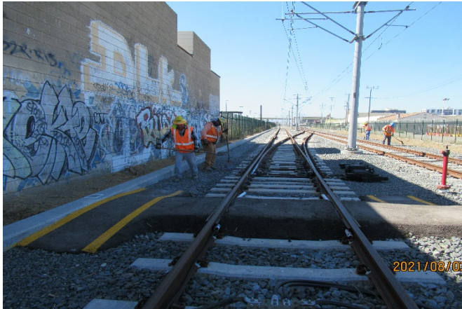
AVIATION STATION – NB track near STA 103+10 Segment A, adding & dressing walkway ballast on right side shoulder
