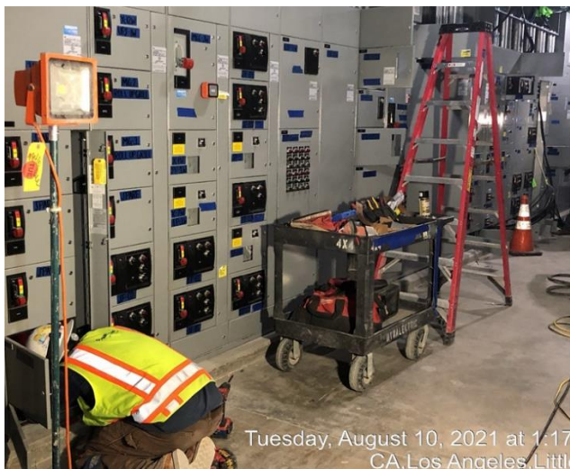
Tuesday, August 10, 2021 at 1:17 CA, Los Angeles, Little 1st/Central Auxiliary Power Room
