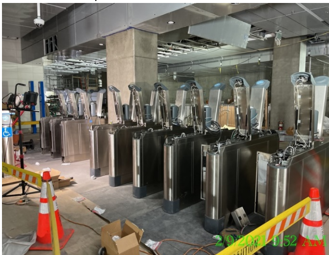
EXPO STATION – Continue setting, drilling and anchoring the fare gate turnstiles at the Paid & Free Area.
