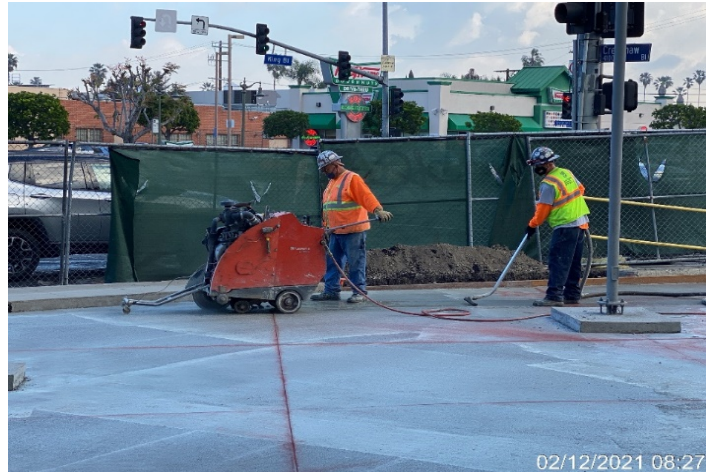
MLK STATION – Saw cutting control joints in preparation for support slab and brick paver installation at the north end area.
