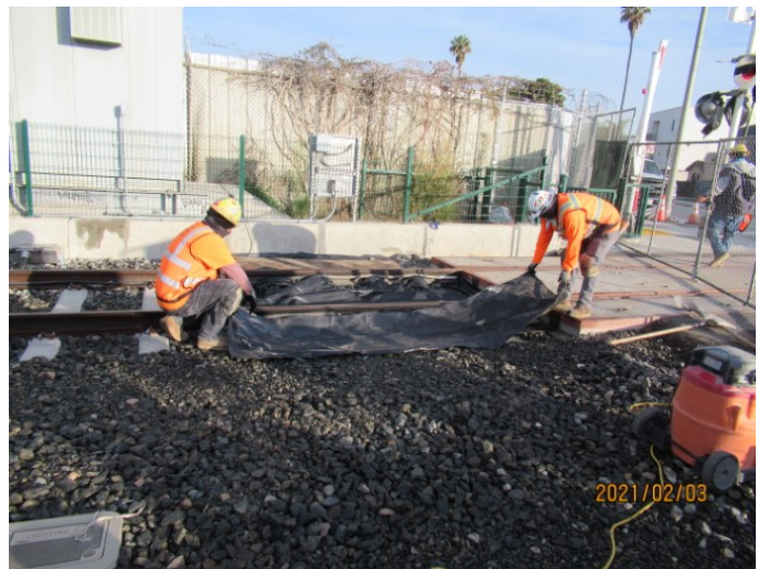
BRYNHURST AVE - WSCC at Brynhurst Ave SB track on south side STA 272+12 covering ballast after cleaning has been completed for BIM 360 number 000620 rework (looking west).
